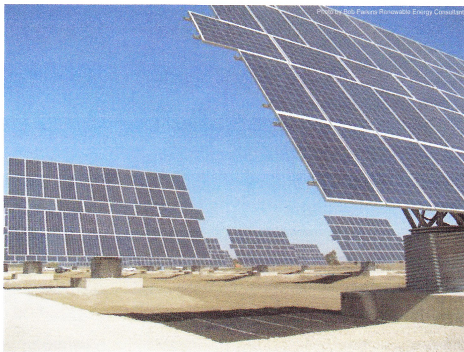
A large-scale system using double axis trackers to maximize energy generation. Changes due to environmental restrictions: The trackers were elevated with dirt mounds and concrete piers to avoid flood potential; the construction cycle was shortened because of endangered species.
